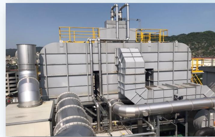
蓄熱式焚化爐(RTO Type) Regenerative Thermal Oxidizer
